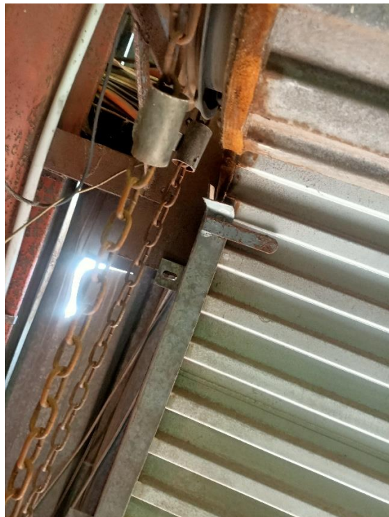
Nylofelt rusting off
