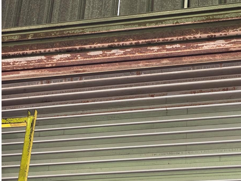
Extensive corrosion to curtain
