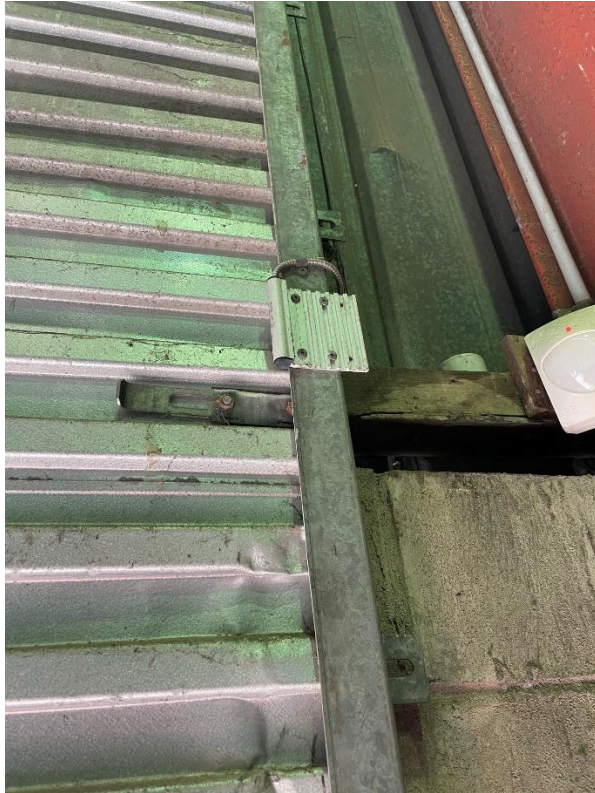
Accessories attached to door i.e. alarm system
