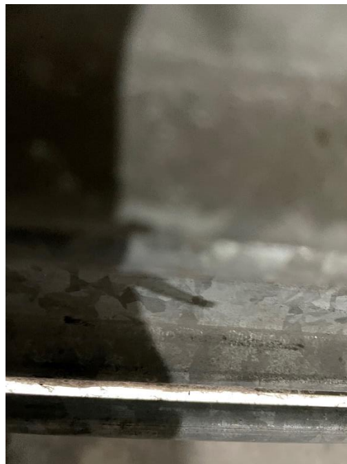
Slats severely damaged. They are pulling apart
