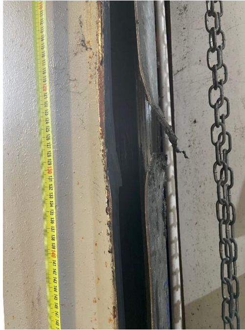
Severe damage to guide
