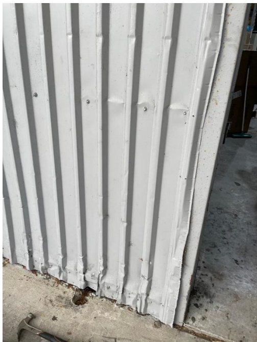
Slat door had been painted same colour as building
