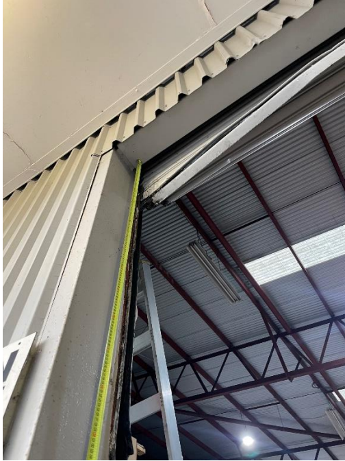
Door opening height – not quite to drum
