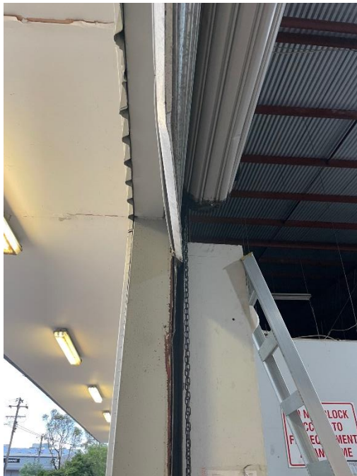
Bottom of shutter door – severely bent. Picture also shows drum location in relation to door opening.
