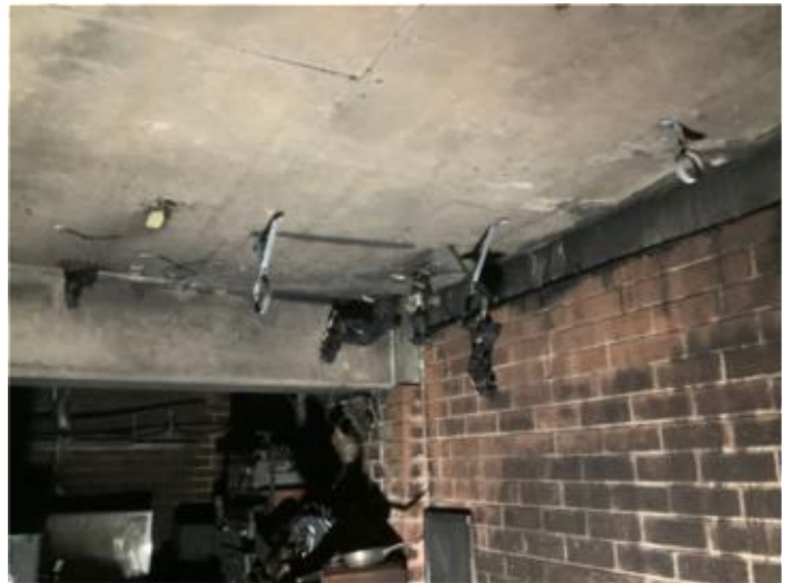
fire damaged aerial water, drainage and gas services located in Unit 7 garages
