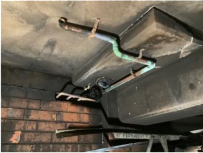
fire damaged aerial water, drainage and gas services located in Unit 7 garages
