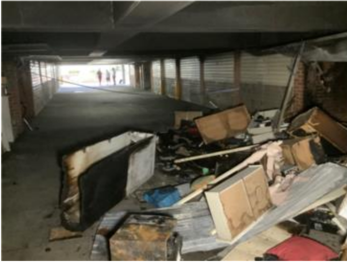
Basement carpark - fire damage & debris
