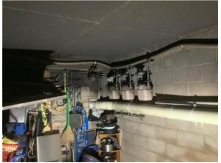
overview gas meters adjacent to unit 7 garages
