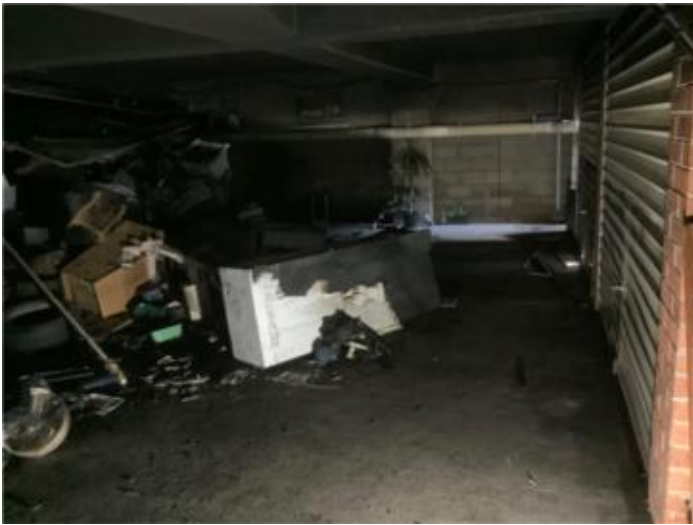
Basement carpark - fire damage & debris
