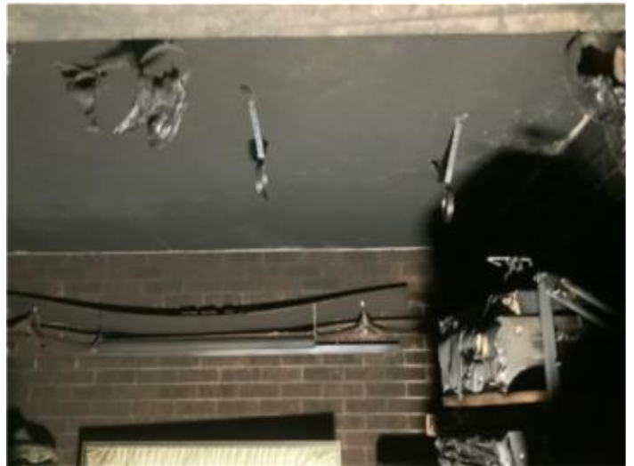
fire damaged aerial water, drainage and gas services located in Unit 7 garages
