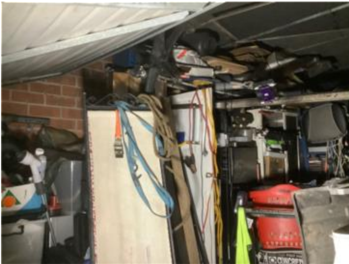
fire damaged aerial water, drainage and gas services located in Unit 7 garages
