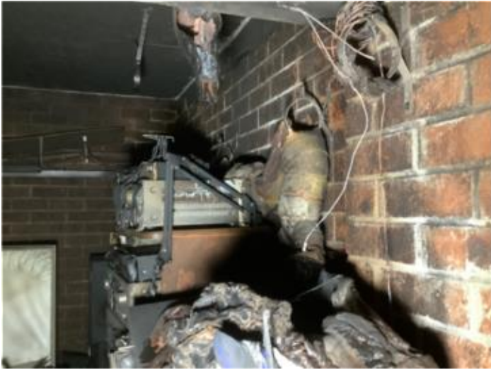
fire damaged aerial water, drainage and gas services located in Unit 7 garages
