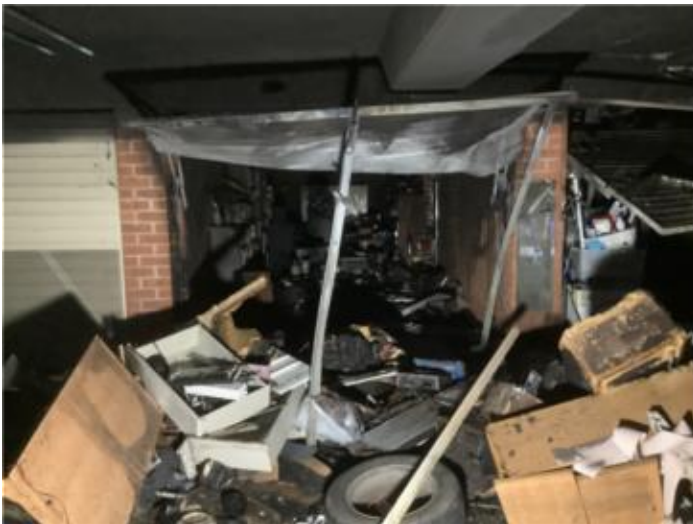
Basement carpark - fire damage & debris in Unit 7 lock up garage garage space
