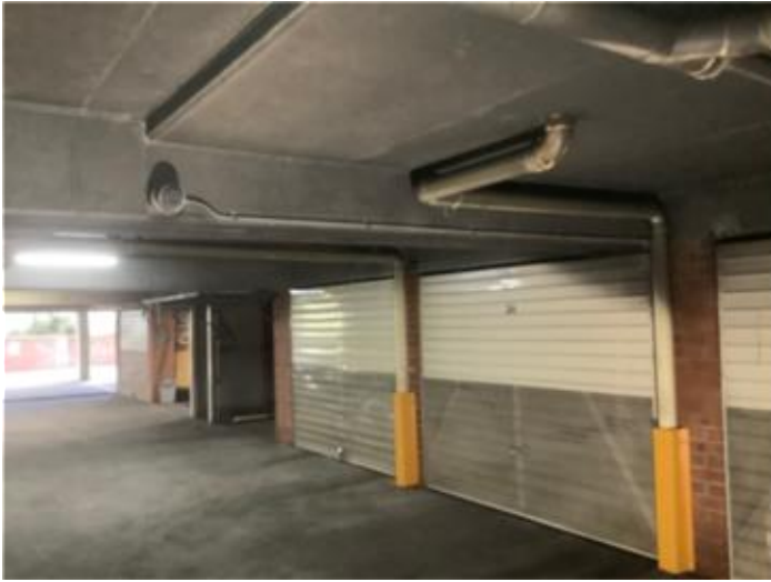
fire damaged CCTV unit mounted on concrete beam adjacent unit 10 garage
