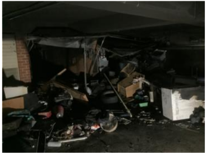
Basement carpark - fire damage & debris
