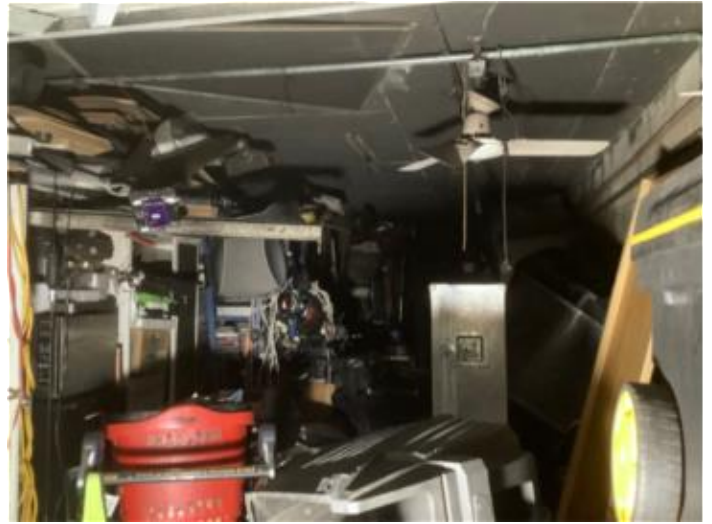
fire damaged aerial water, drainage and gas services located in Unit 7 garages
