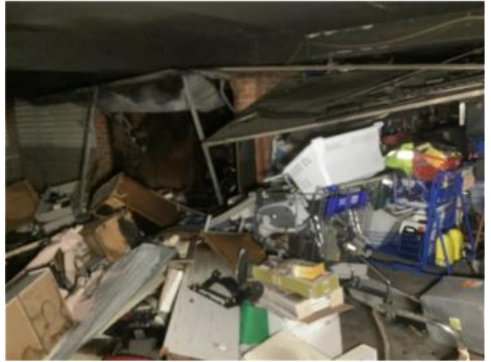
Basement carpark - fire damage & debris
