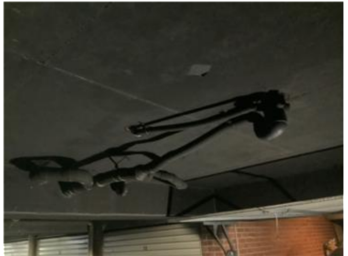
aerial drainage adjacent unit 10 garage and away from unit 7 garage fire
