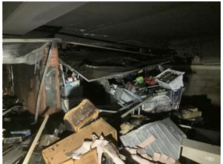
Basement carpark - fire damage & debris in Unit 7 lock up garage garage space
